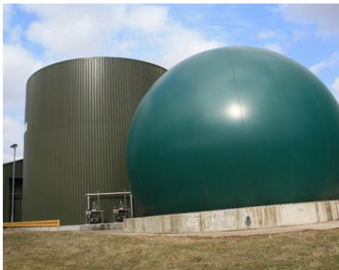
The anaerobic digestion plant using exclusively out-grade crop handled on site
